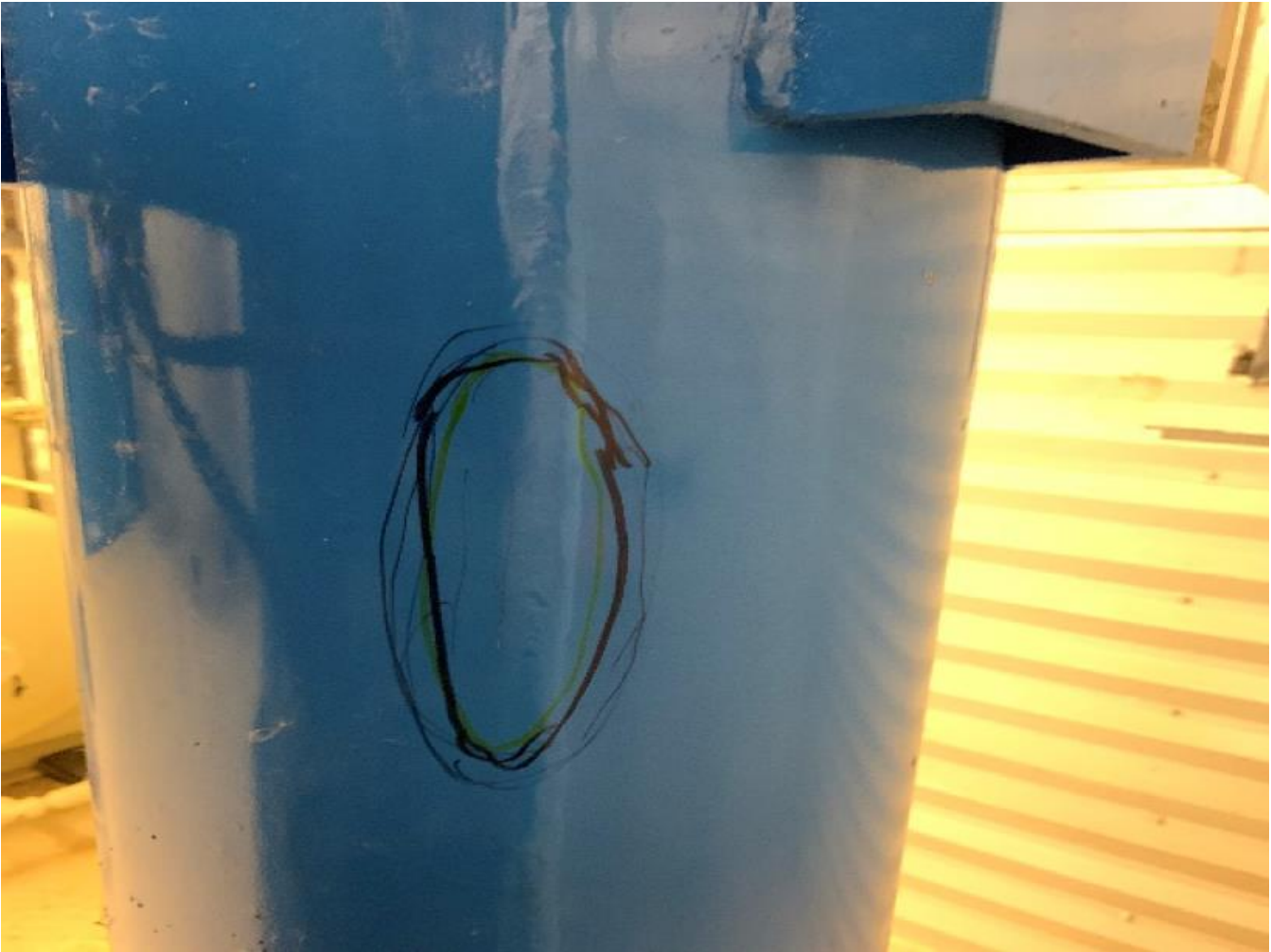
Area of crack along vertical weld seam.
