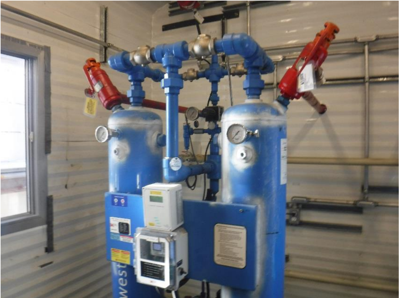
Air dryer overview.
