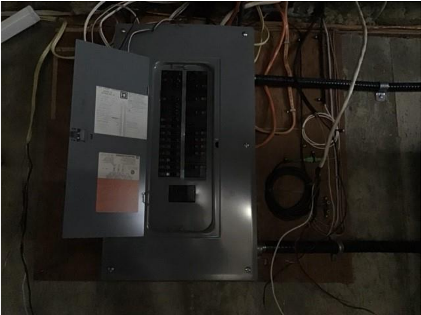
Main dwelling panelboard, installed on basement level
