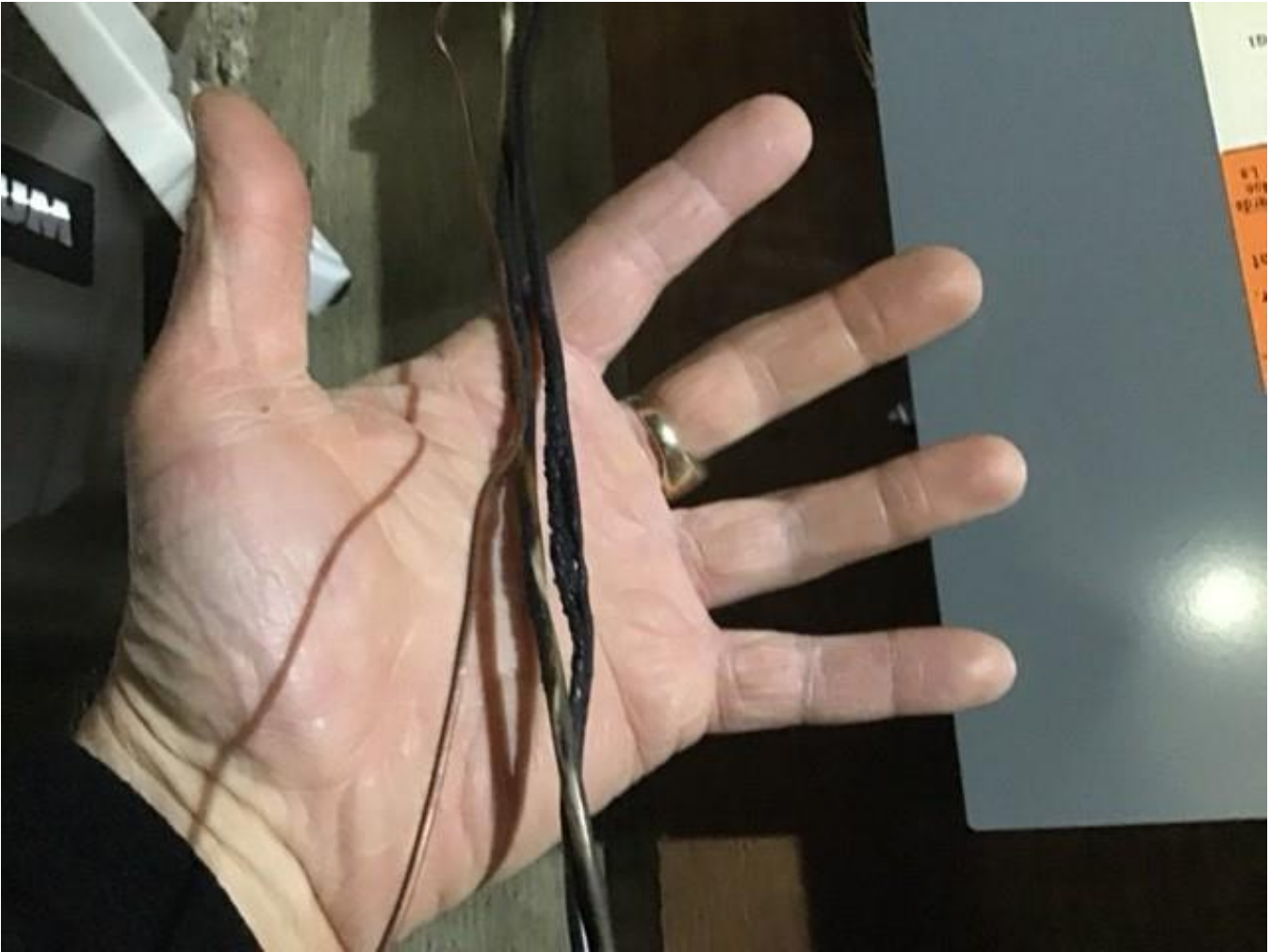
Burnt branch wiring conductor insulation
