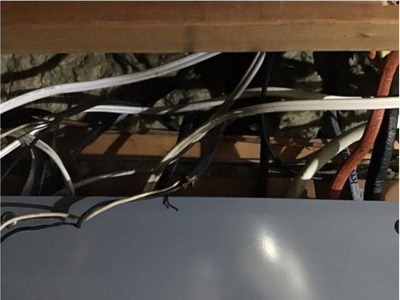
Burnt branch wiring cable insulation above panelboard
