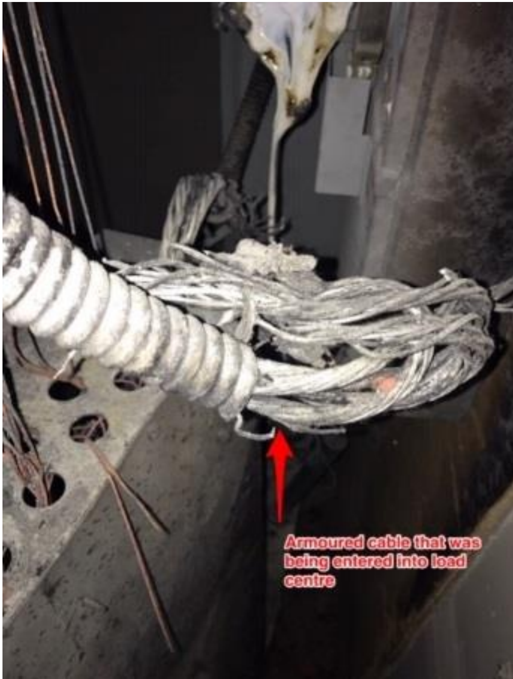
Photograph 2. Armoured cable that was being entered into load centre
