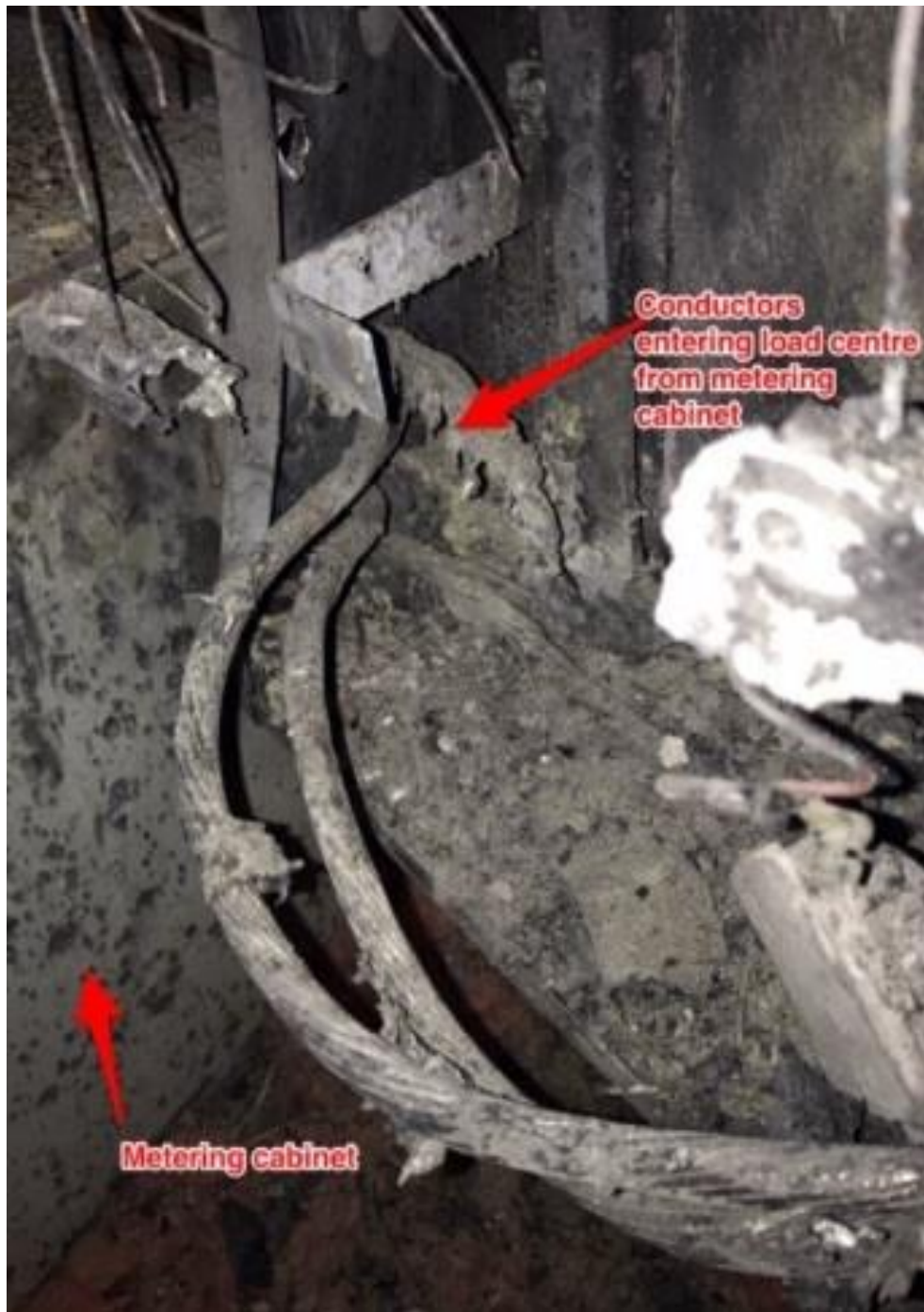
Photograph 3. Meter cabinet location and associated conductors entering load centre
