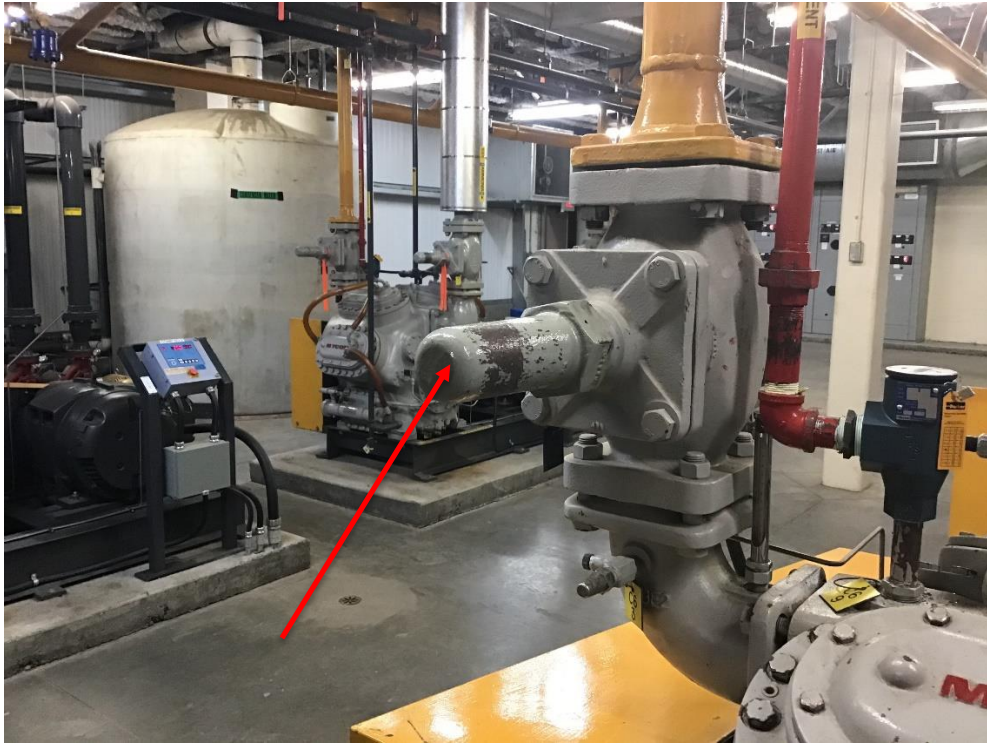
Compressor Number 6 Discharge Valve with valve stem bonnet (bonnet protects valve from potential external damage such as forklifts or other potential damage)
