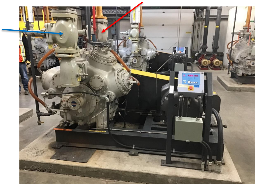
Above-Compressor Number 6 Overview: Blue arrow is inlet suction valve
