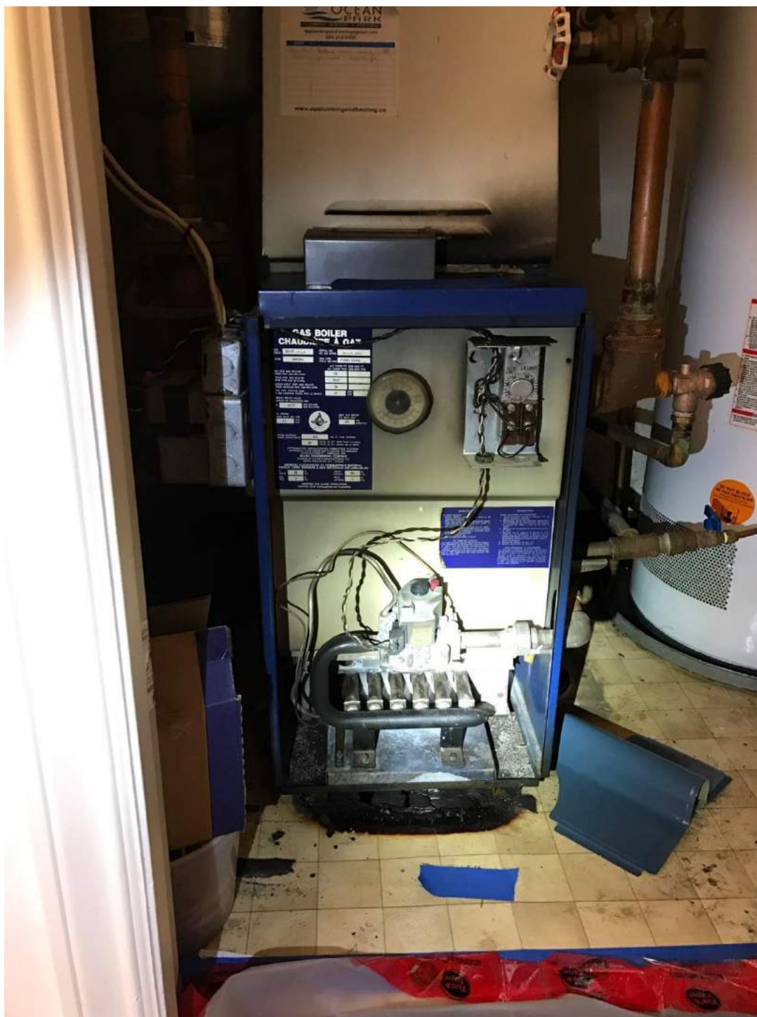
Figure 1: Front of boiler after fire.
