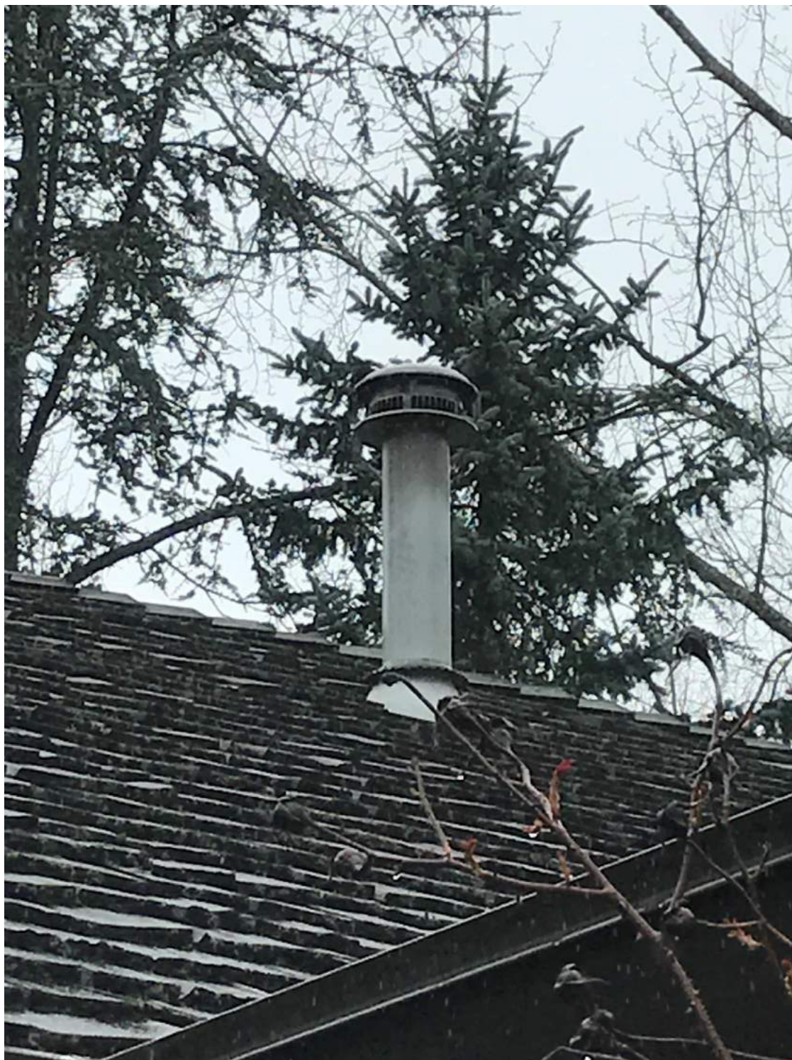
Figure 7: Roof termination for boiler, showing sooting beyond what would be expected from this type of appliance if it were burning properly.
