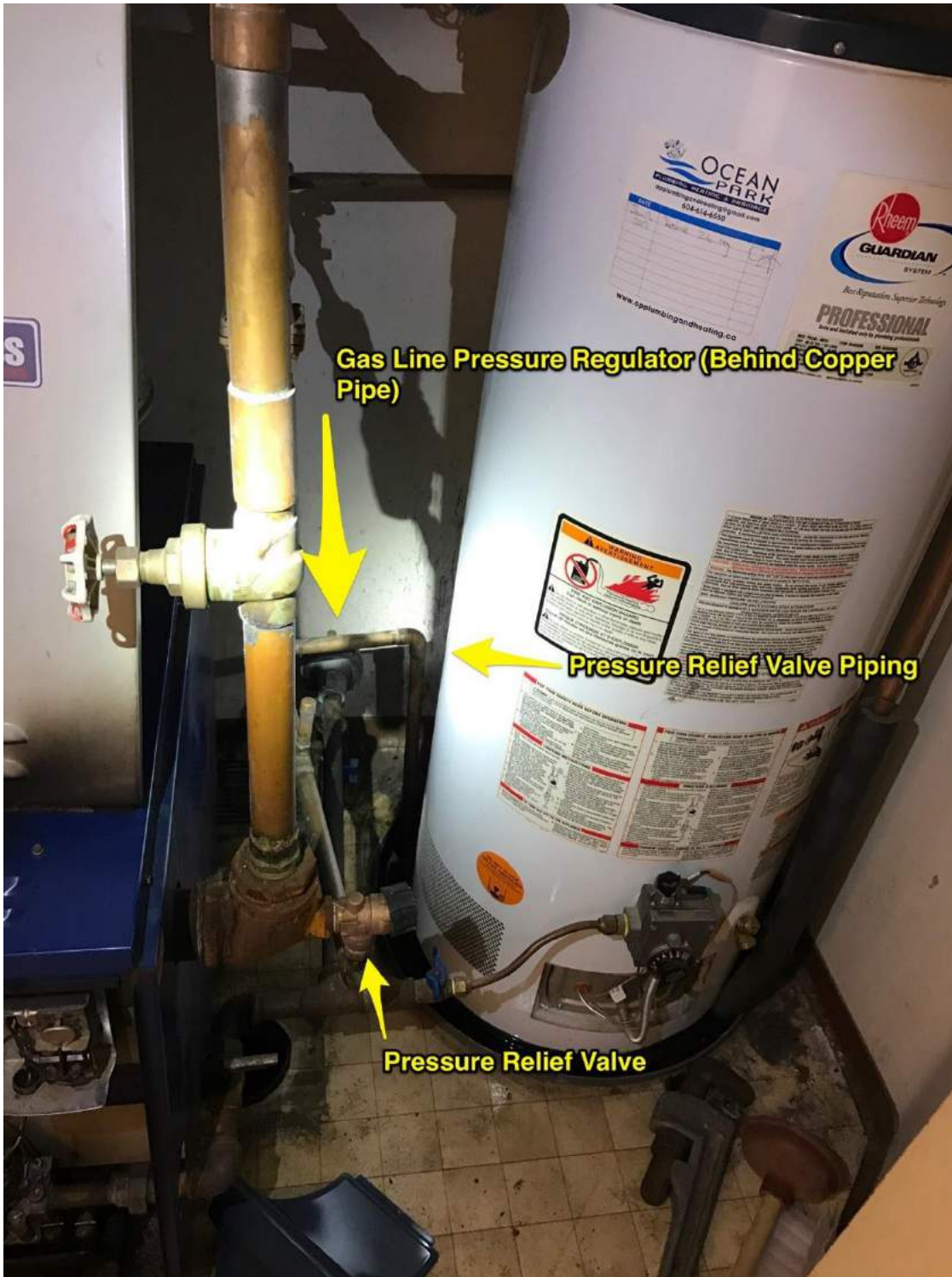
Figure 4: Pressure relief piping, and gas line pressure regulator.
