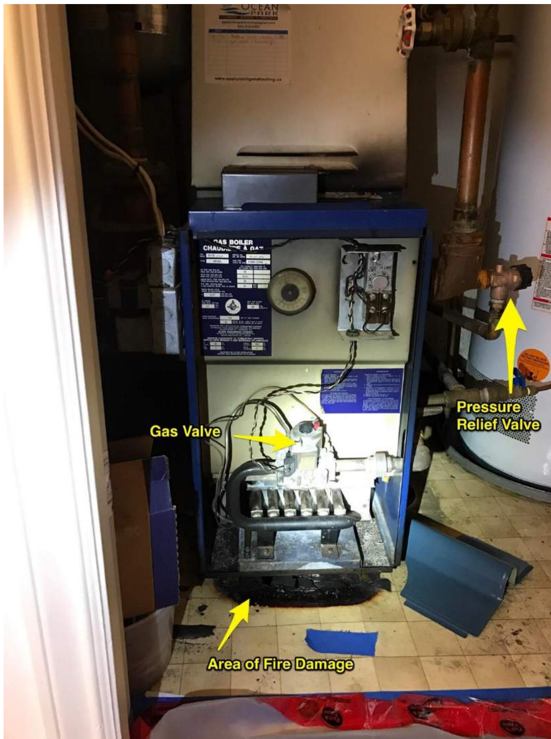
Figure 3: Front of boiler annotated to show components and fire damage.
