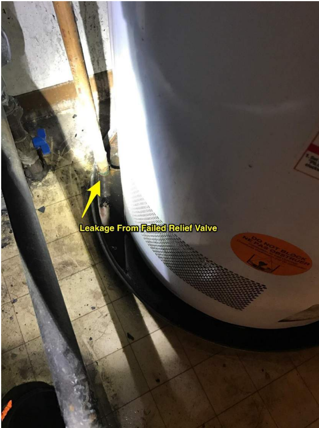
Figure 5: Discharge of relief piping showing leakage.
