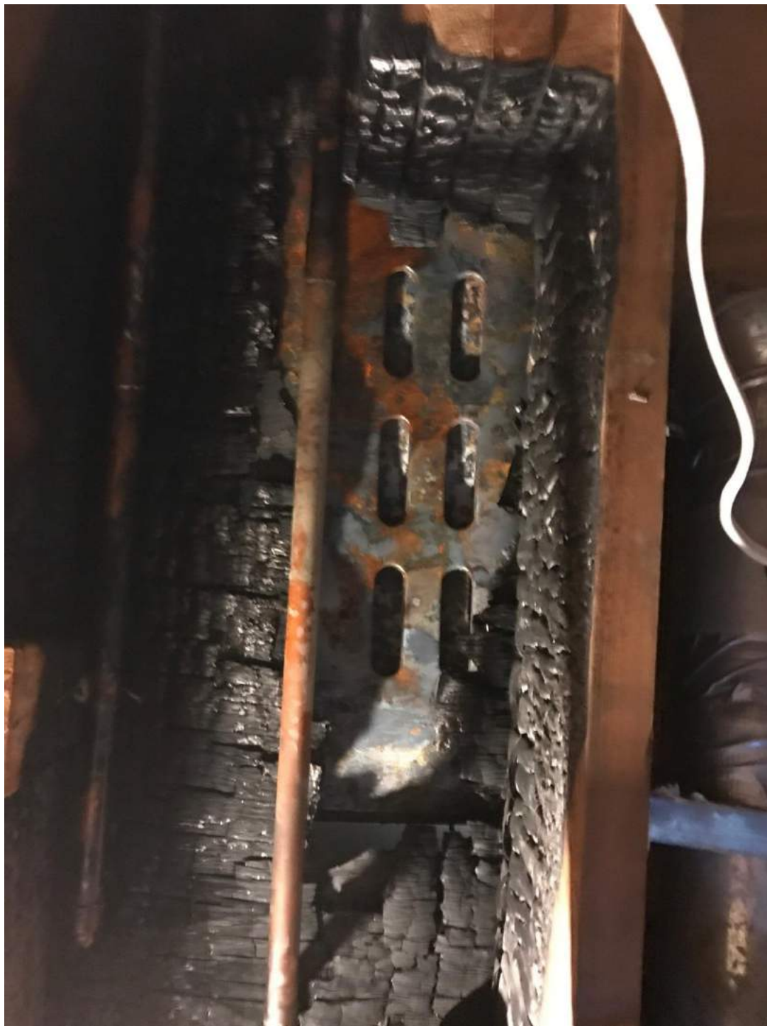
Figure 8: Fire damage below boiler.
